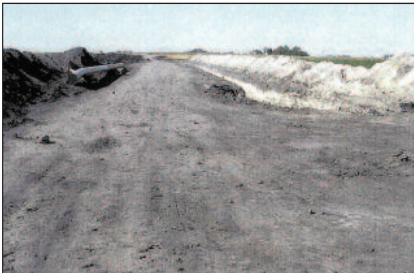
Construction road through farm field creates soil compaction.
